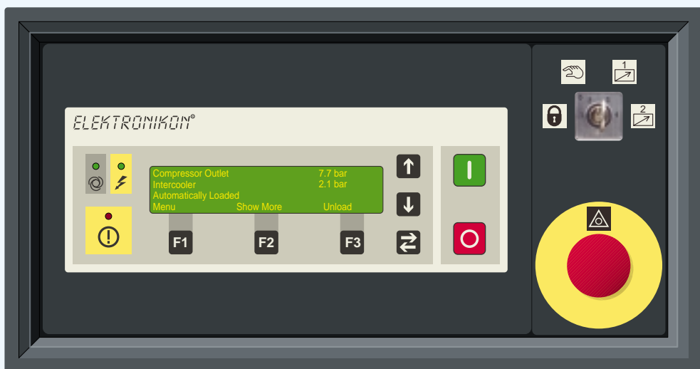
A user-friendly monitoring panel shows all the operating parameters for the compressor, for example, pressure and temperatures, with data logically grouped for direct read-off.
